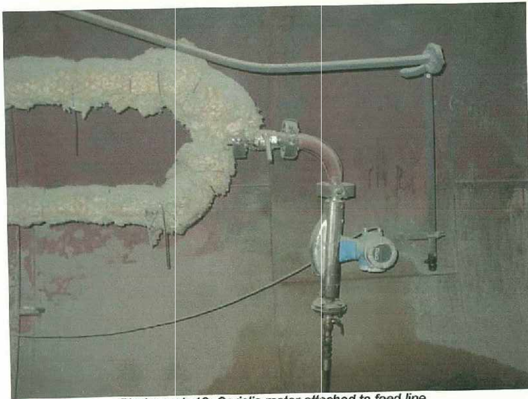
Photograph 18: Coriolis meter attached to feed line
