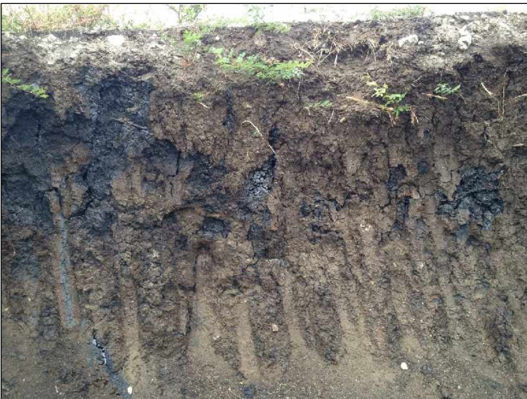
Plate 9. View of tar residue seeping out of pit wall on Tar Dam B (South)
