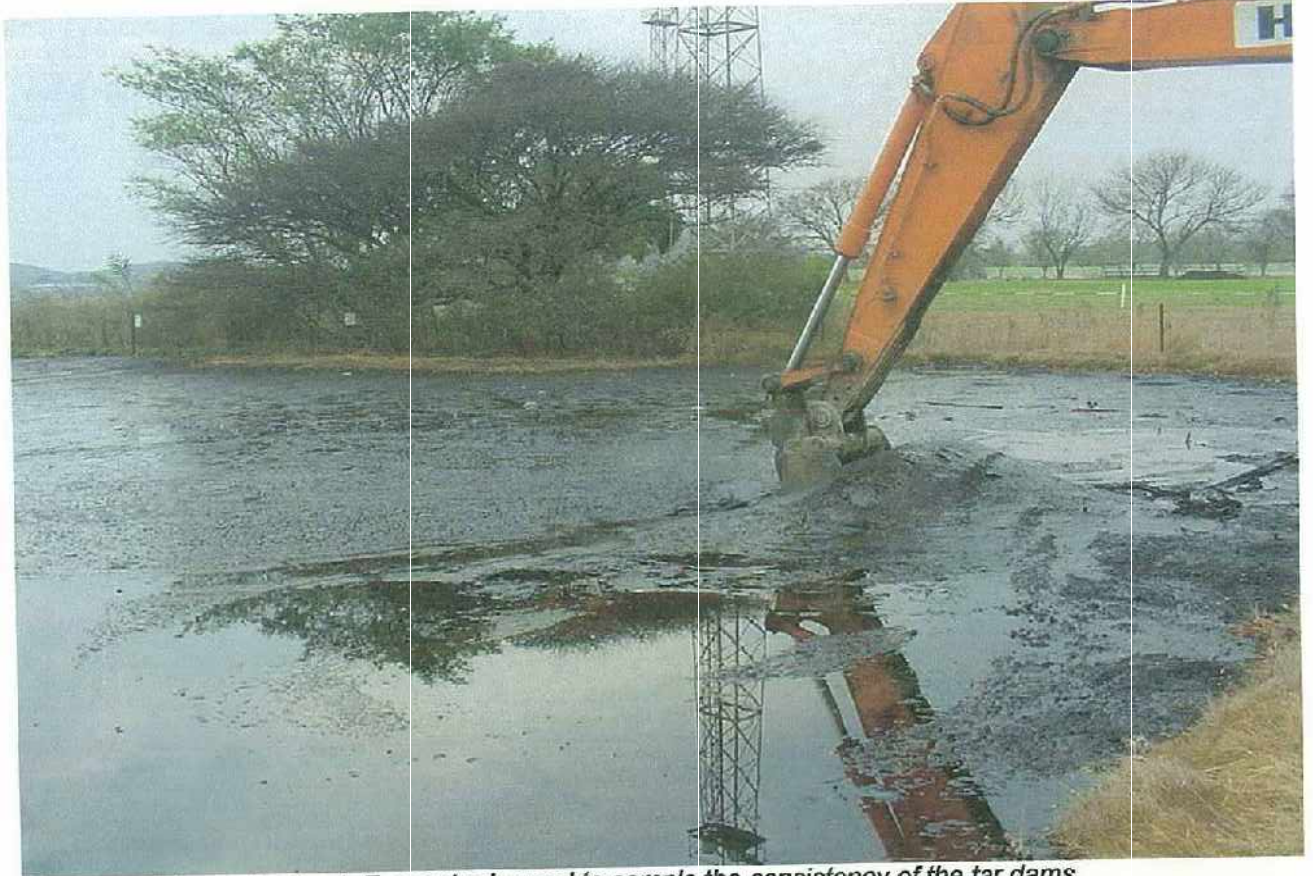
Photographs 1 – 4: Excavator is used to sample the consistency of the tar dams
