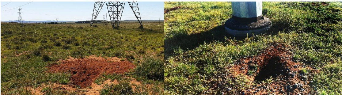
Figure 7: Active burrows in close proximity to power line infrastructure, indicating that the presence of these structures did not deter burrowing animals from the site. Springhare potentially take advantage of the disturbed soil and short grasses surrounding the pylons.
