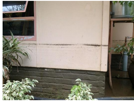
Water level mark on house
