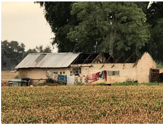
Staff housing roof ripped away
