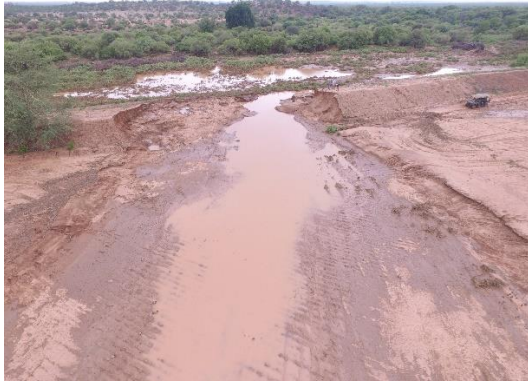
Bund wall collapsed by water force
