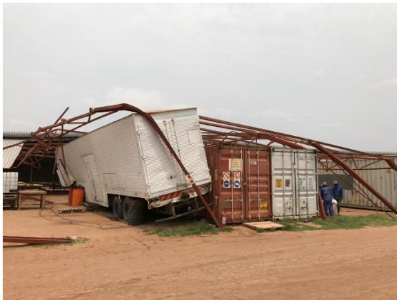
Collapsed shed on equipment
