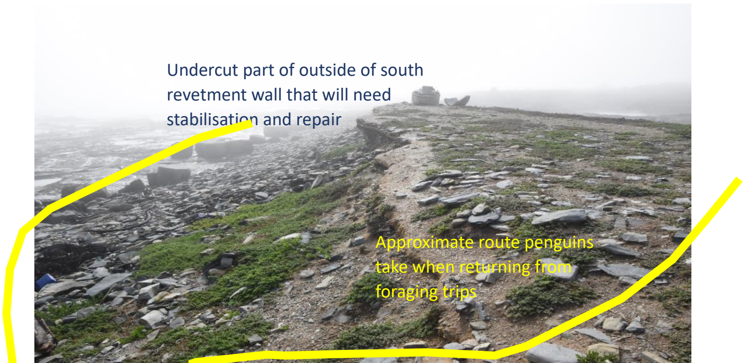
Figure 2 photograph taken at the top of the south revetment wall in early June 2021 overlaid with a sketch showing the route penguins returning from the sea take to reach the foot of the wall and then climb over it. The damaged (undercut) part of this wall can be seen top centre.
