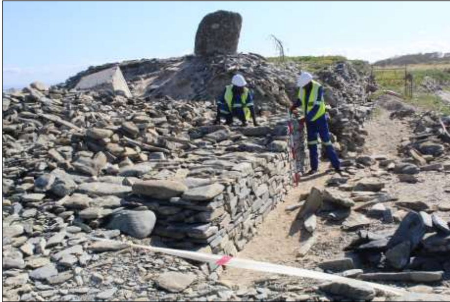
Figure 7: Sand load placed in the core of the wall can be seen below the concrete cube in the background. The recommended packing of the core excluding the sand can between two concrete cubes in the foreground.
