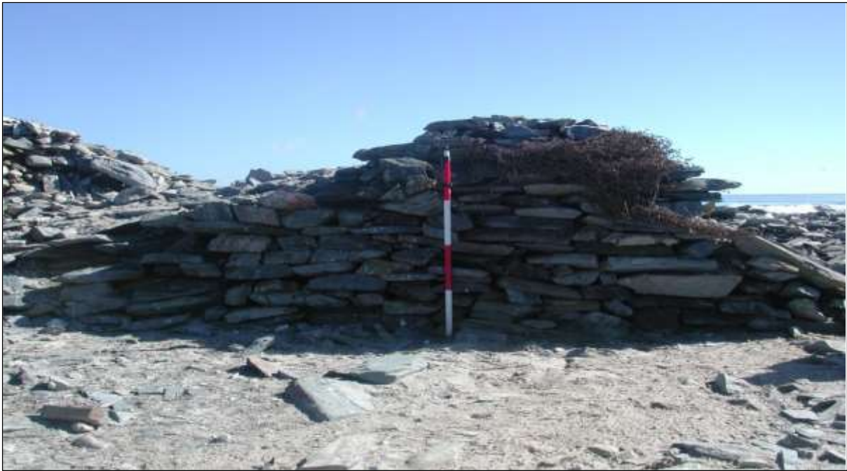
Figure 6: This wall was standing in 2004 in the section that was washed away in 2011. It shows the frequent use of façade stones with long faces. There is poor structural coherence, i.e. bonding between the façade and the core (Matenga 2004, page ix).
