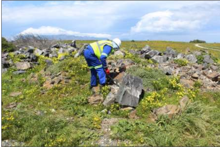
Figure 9: Stockpile of raw stone to be broken and used for the construction of the BSQW.
