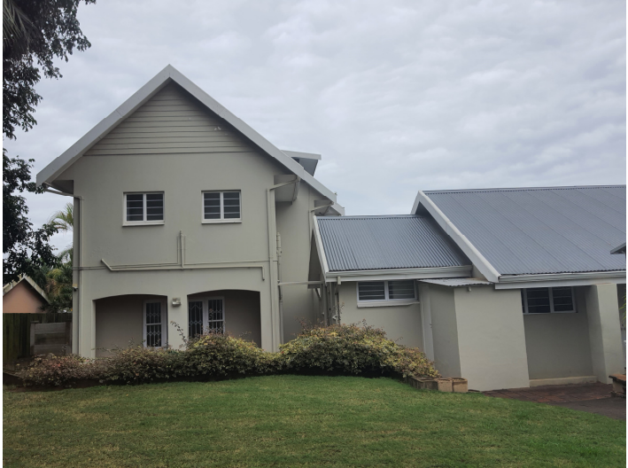
PART NE ELEVATION SHOWING THE DOUBLE STOREY FACADE ON WHICH THE PROPOSED ADDITIONS WILL BE LINKED – (BEFORE)
