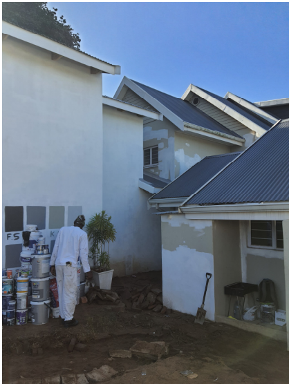
MORE OF SW ELEVATION SHOWING THE LINK BETWEEN THE OLD AND THE NEW
