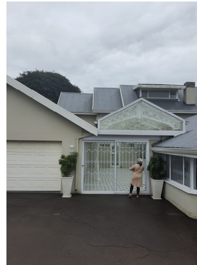
PART SW ELEVATION SHOWING THE ROOVES TO BE AFFECTED IN THE BACKGROUND
