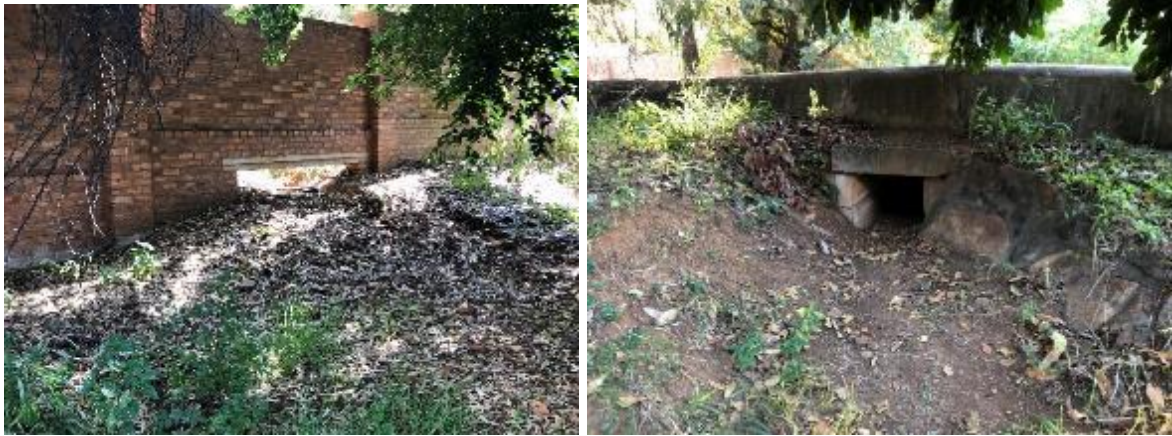
Figure 5.11: The opening in the boundary wall to Erf 348 and the culvert under the unnamed road.
