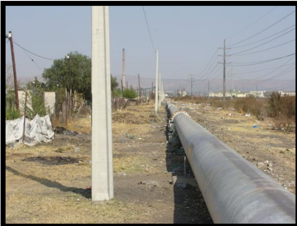
Figure 11: Route along the existing compressed air pipeline, where the additional pipeline is being proposed.
