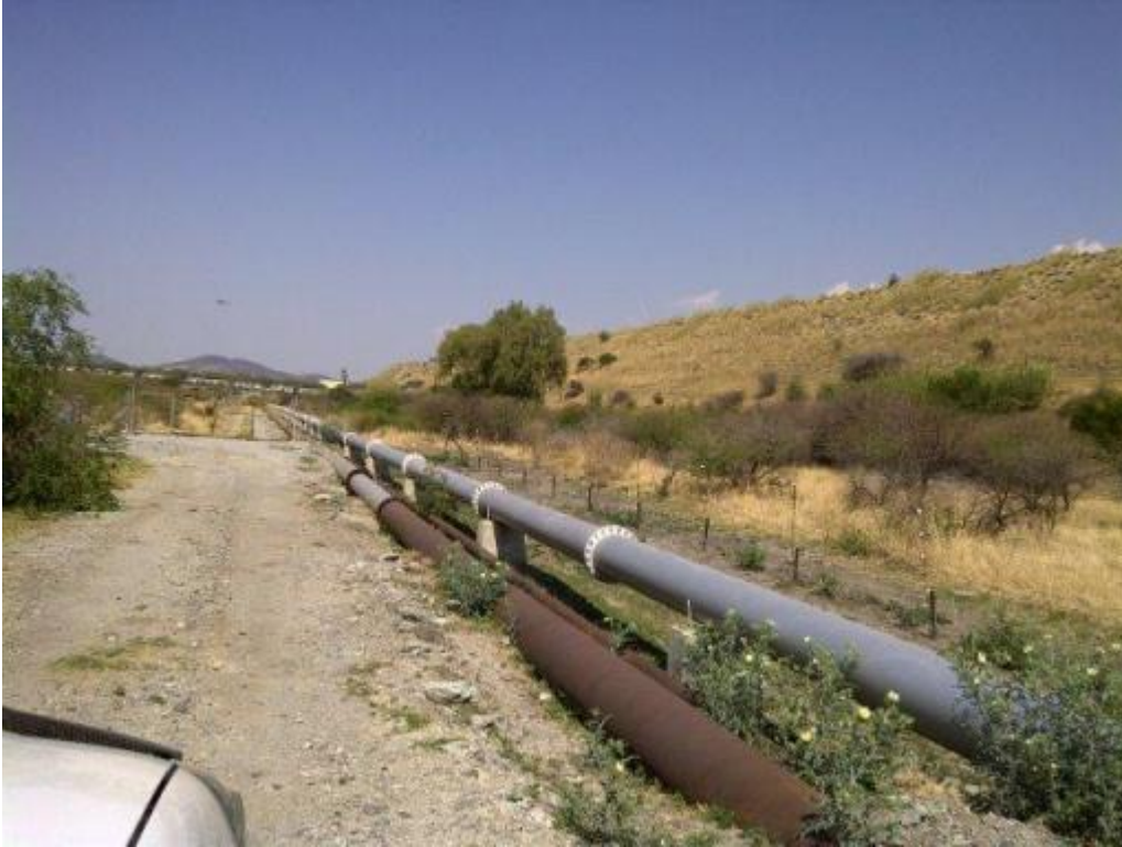
Figure 12: Example of overland pipeline
