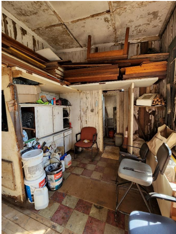
Image 9, 10 and 11: Damage to internal walls and Ceilings
