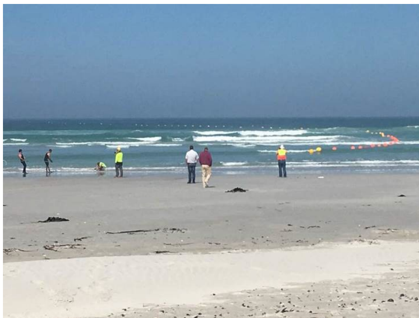
Figure 7 Example of a cable being guided to shore by divers and small boats
