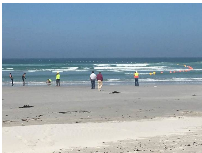
Figure 7 Example of a cable being guided to shore by divers and small boats
