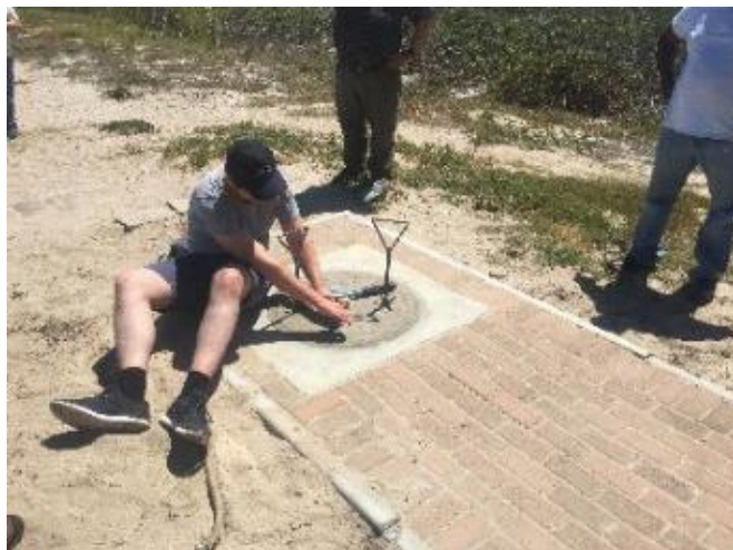
Figure 9 ACE BMH which will be used for the landing of the 2AFRICA (East) cable landing.
