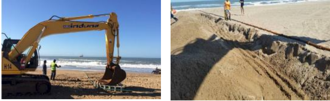
Plate 7 Landing of the cable on shore. Similar works will be undertaken for the landing of the 2AFRICA/GERA (East) Cable System
