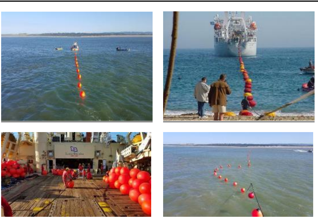
Plate 8 Bringing the cable to shore from the cable laying vessel. Cable is buoyed off and pulled to shore with smaller vessels.
