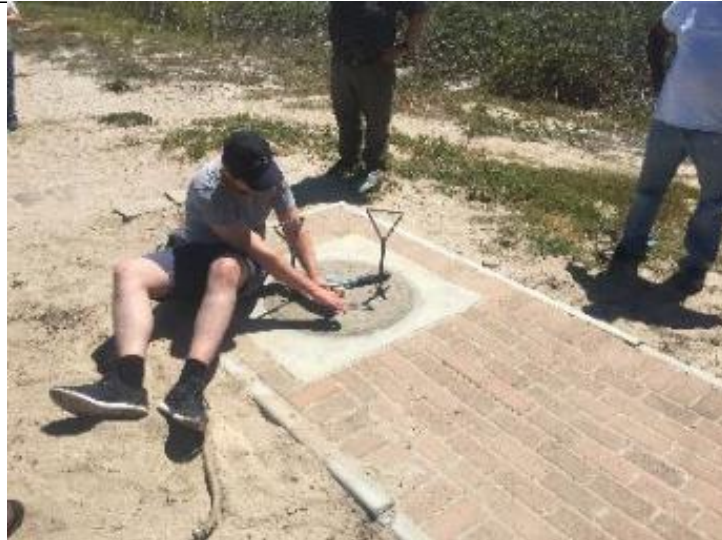
Figure 8 Example of a BMH for the landing of the 2AFRICA (East) cable landing.
