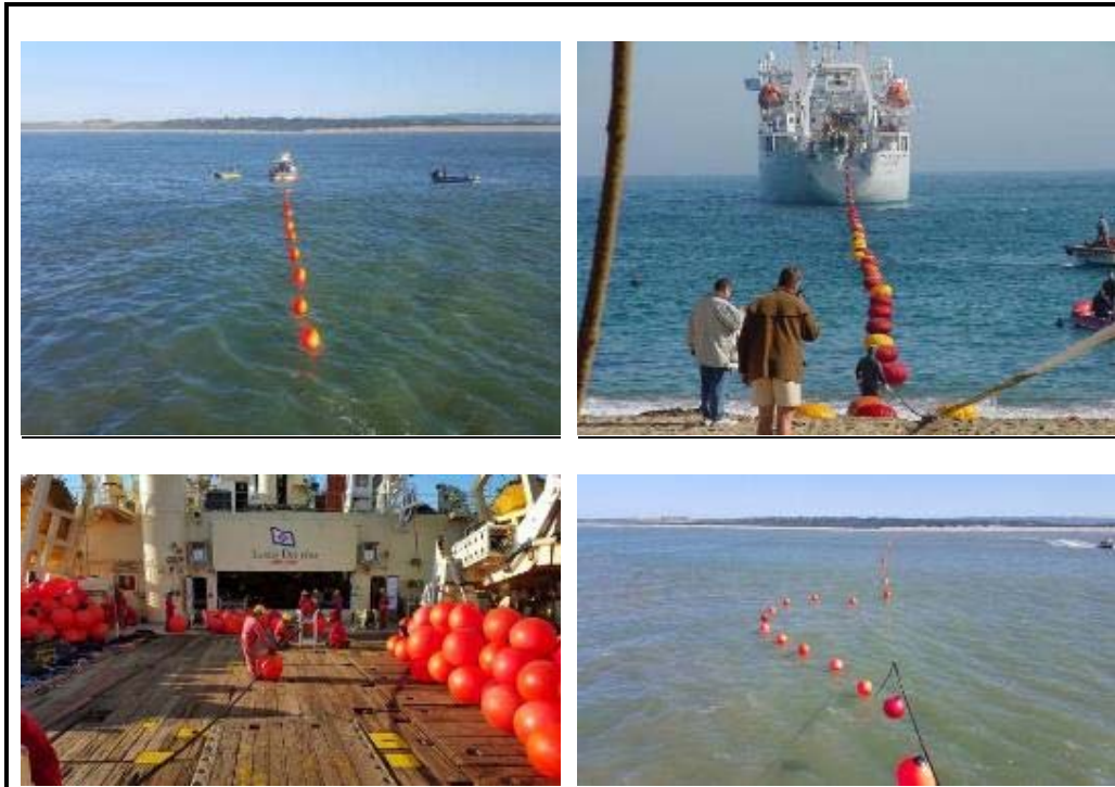
Plate 8 Bringing the cable to shore from the cable laying vessel. Cable is buoyed off and pulled to shore with smaller vessels
