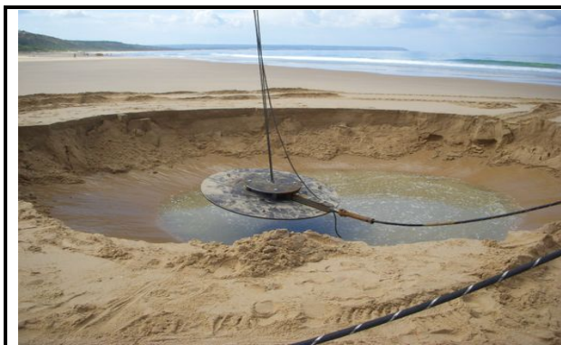
Plate 9 Example of a sea earth plate (System Earth) which must be installed in saturated soil
