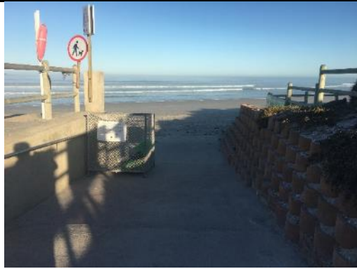
Beach access path under which the WACS pipe conduit to the beach is buried
