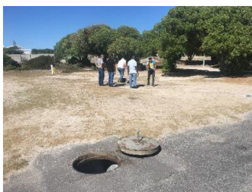
Existing WACS man hole on the front haul alignment
