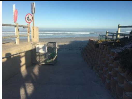
Beach access path under which the WACS pipe conduit to the beach is buried
