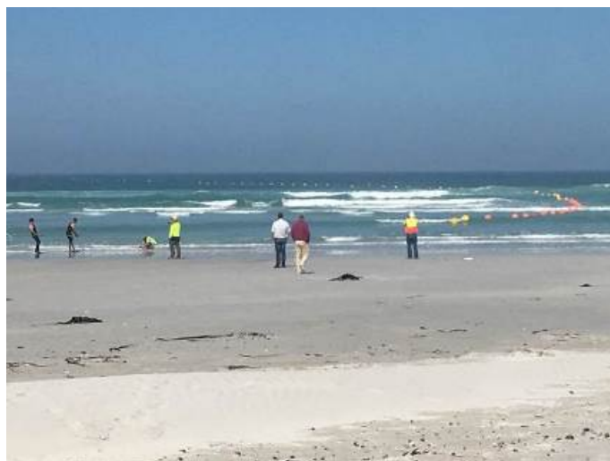
Figure 6 Example of a cable being guided to shore by divers and small boats
