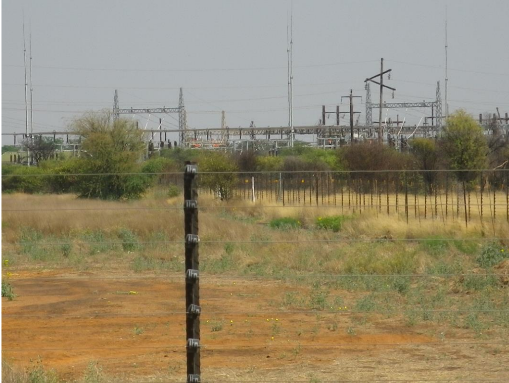
Photo 1: View of the Klipkop substation from where the proposed powerline will start.
