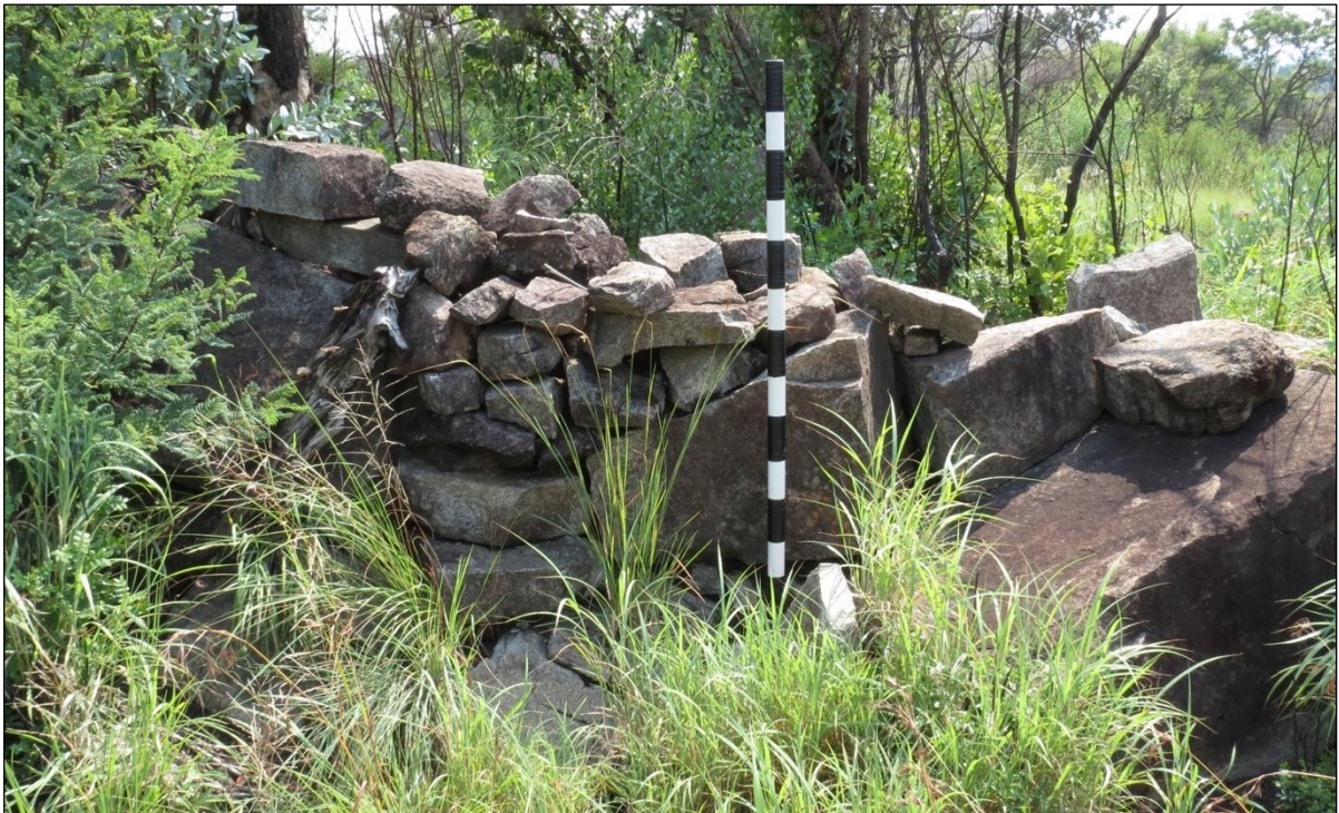
Figure 90 – Side view of a section of the stone packed wall at feature DBAP 19B. Scale in 10cm increments.
