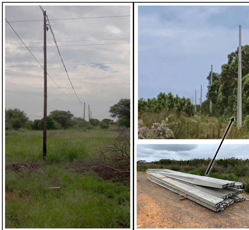
Figure 6: Examples of fibre optic cables installed on timber (left) and concrete (right) poles.
