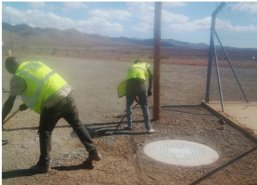
Figure 5: Example of a surface manhole to allow access to the underground fibre optic cable during operations and maintenance.
