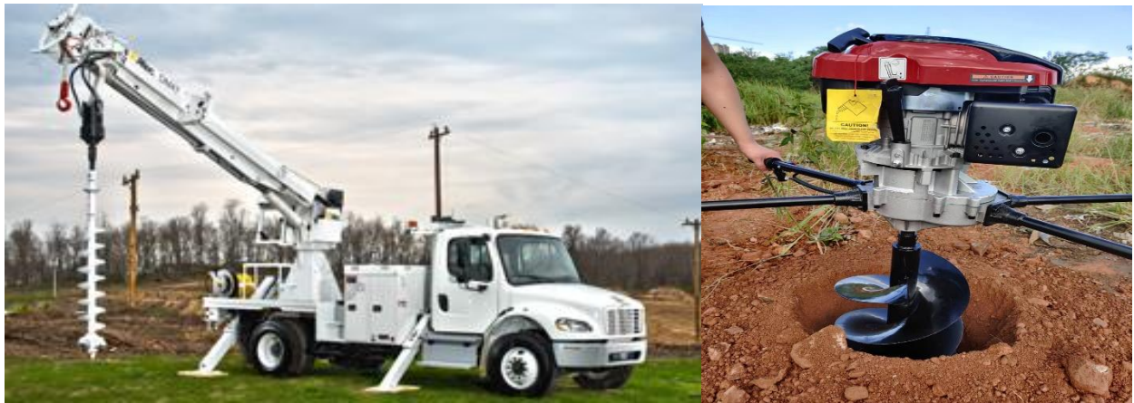
Figure 7: Holes for installing overhead cabling poles will be dug by truck-mounted (left) or hand-held (right) drills.
