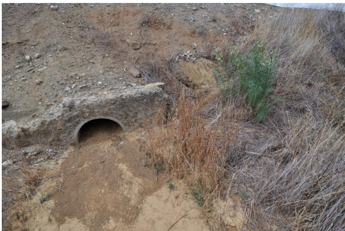
Plate 2: Presently the road crossings impede upstream flows as a result of being undersized thus trapping sediments and becoming blocked.
