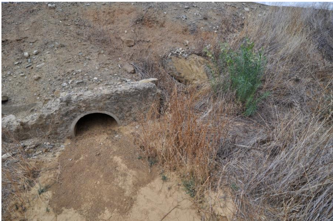
Plate 2: Presently the road crossings impede upstream flows as a result of being undersized thus trapping sediments and becoming blocked.
