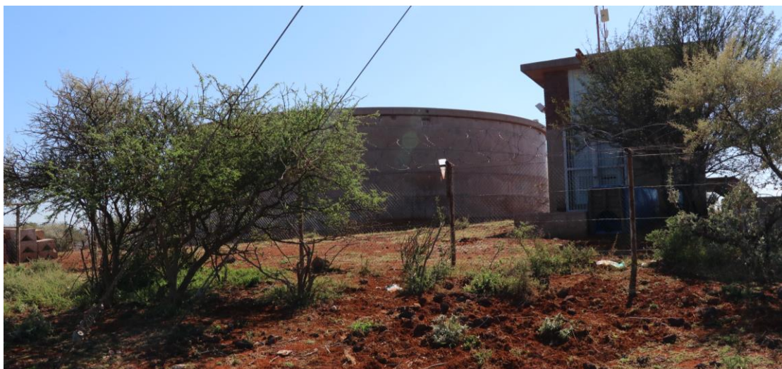
Figure 5: View of the existing reservoir complex on top of the low hill at the eastern end of the pipeline route.
