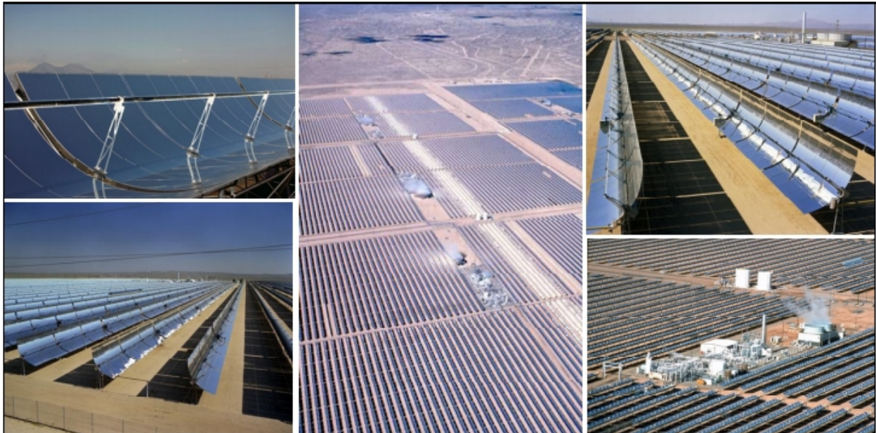
Figure 2.7 CSP parabolic trough plants, Kramer Junction California
