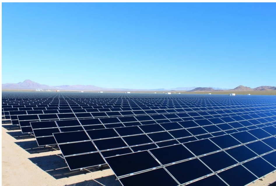
Figure 2.6: Examples of a Photovoltaic facility
