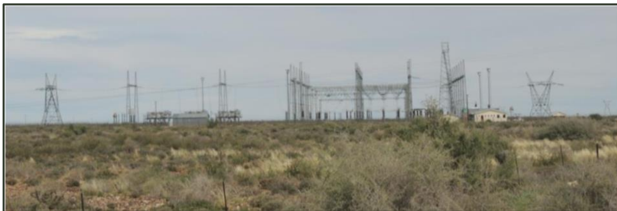
Figure 5-13 View of existing Kronos substation (VRM, 2013)
