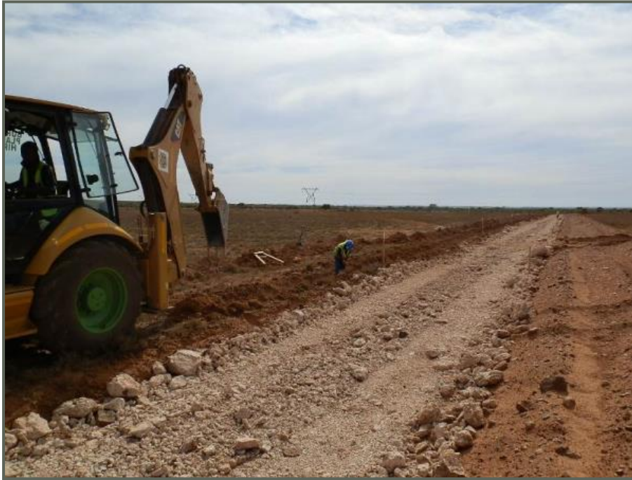
Figure 3-7 Example of a site access road being constructed (image courtesy of SunPower)
