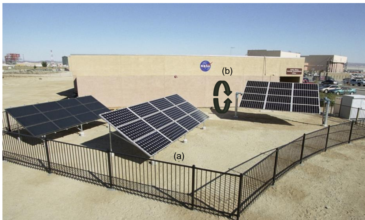
Figure 3-14 Fixed axis tracking system (a) and single axis tracking system (b) (courtesy Mulilo)
