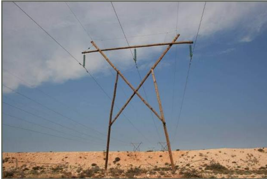
Figure 3-3 Example of an existing 132 kV transmission line (taken 29/09/2011)
