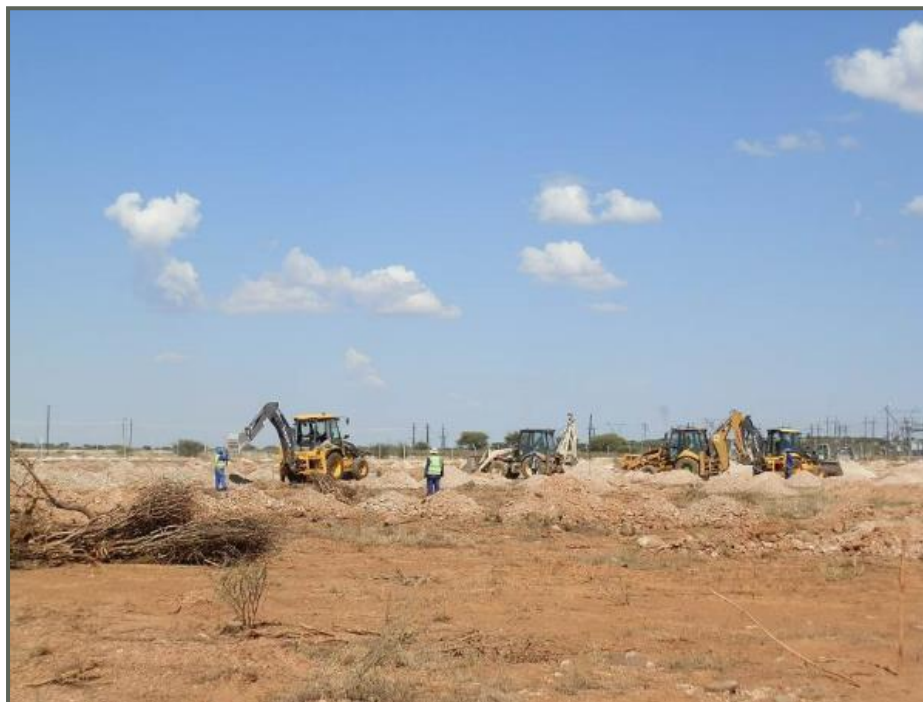
Figure 3-8 Example of a PV site being prepared for construction (image courtesy of SunPower)
