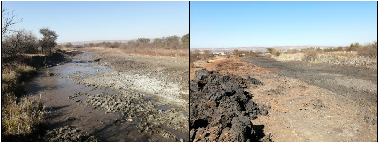
Figure 10. Photographs of construction activity within the Montanaspruit immediately upstream of the project study area.
