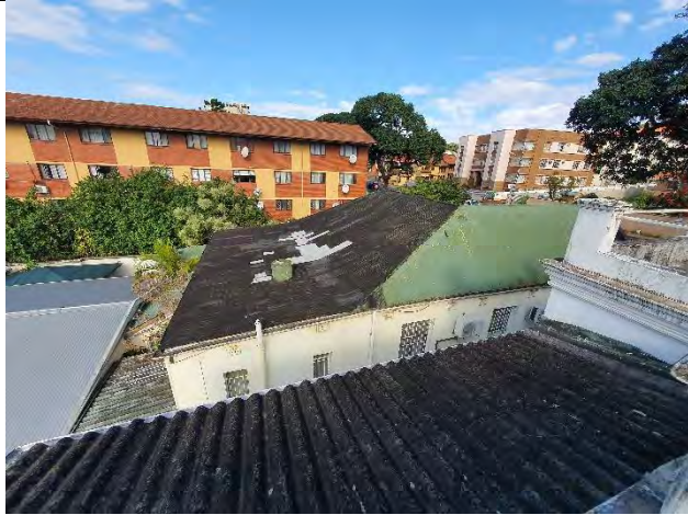
Figure 19: Existing sheeted roof over original dwelling on no. 99 and over the new extension
