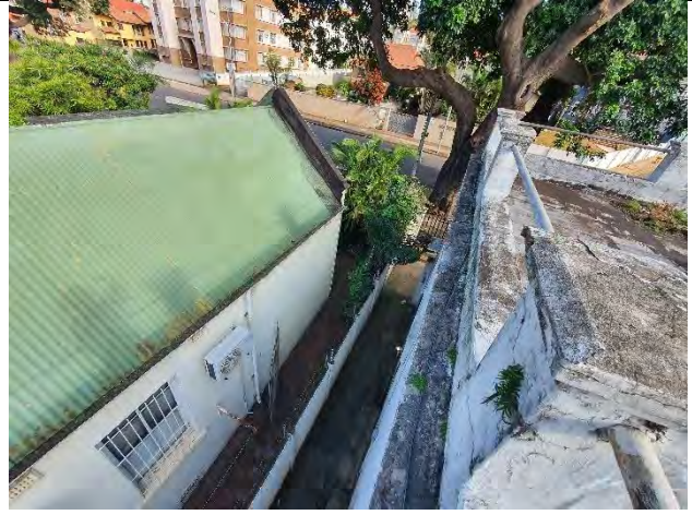
Figure 18: View of roof and side space as seen from the roof of no. 101
