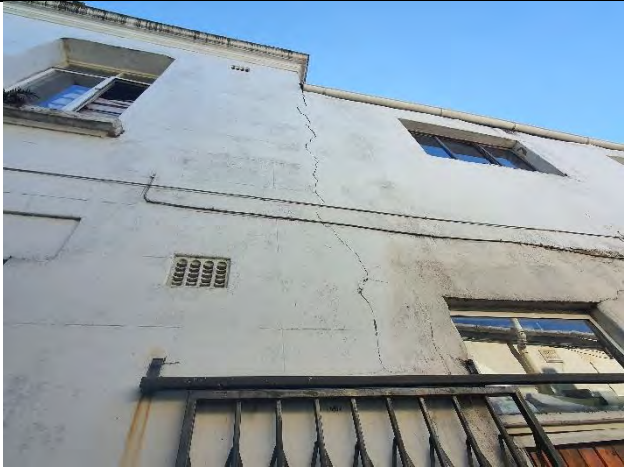
Figure 3.1: Cracks on rear elevation where balcony is enclosed
