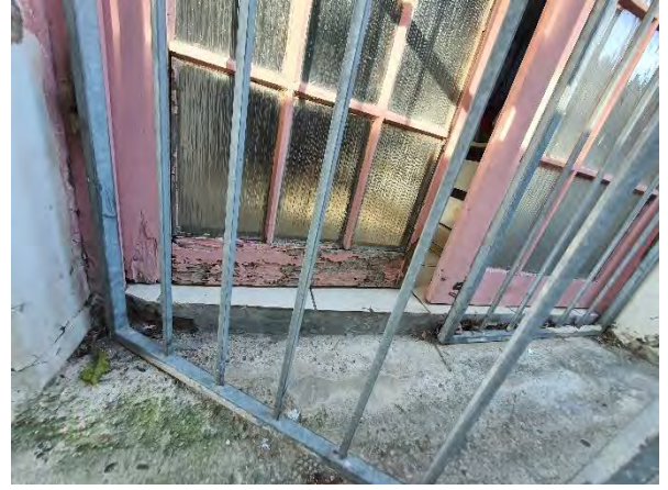
Figure 2.10: Existing door and wooden frames rotted
