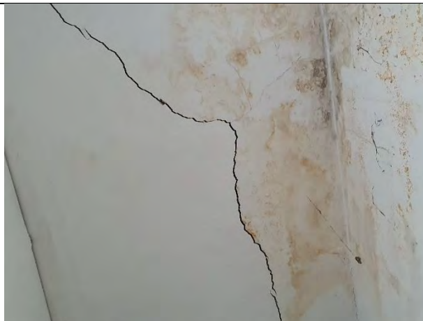
Figure 3.8: Cracks on structural party wall between 105 & 101
