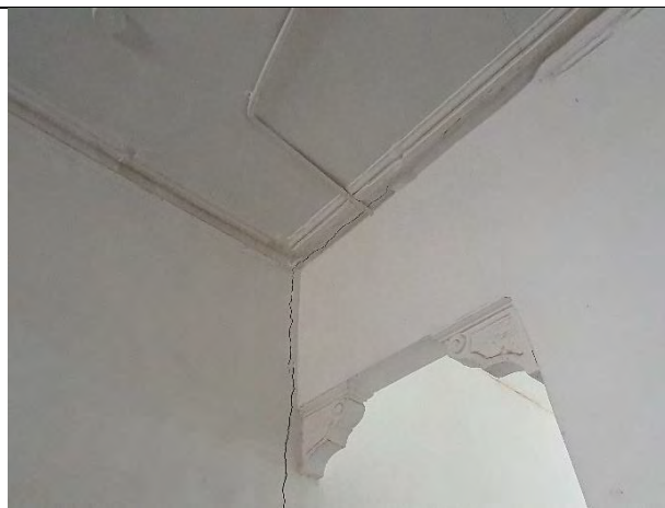
Figure 3.10: Structural cracks to internal walls
