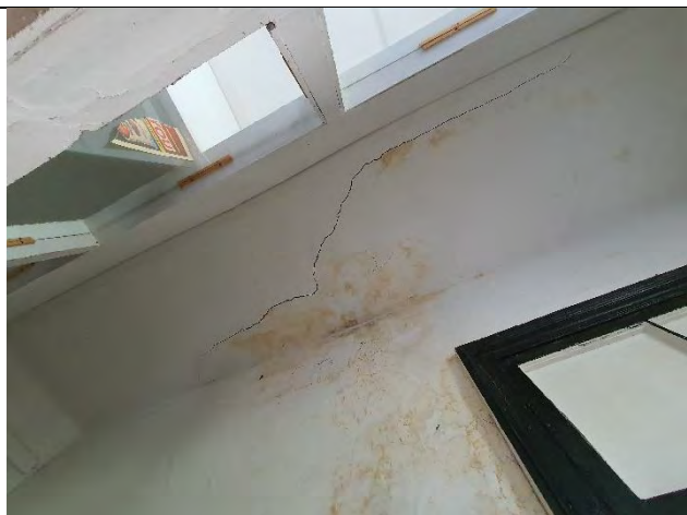
Figure 3.9: Structural cracks to internal walls & slab
