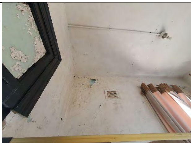
Figure 3.11: Water damage to walls & soffit from roof slab leaks
