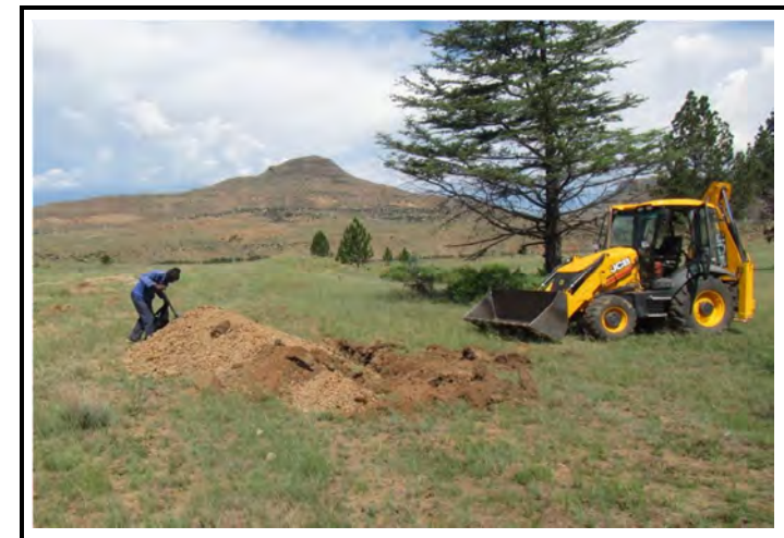
View of potential borrow pit target area - looking down the dyke footprint
