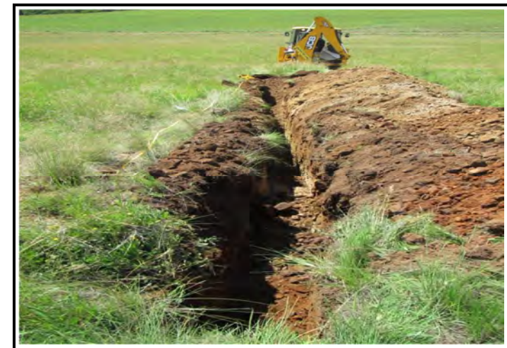
View of trench (15 m long) excavated in potential borrow pit target area to determine width of dyke
