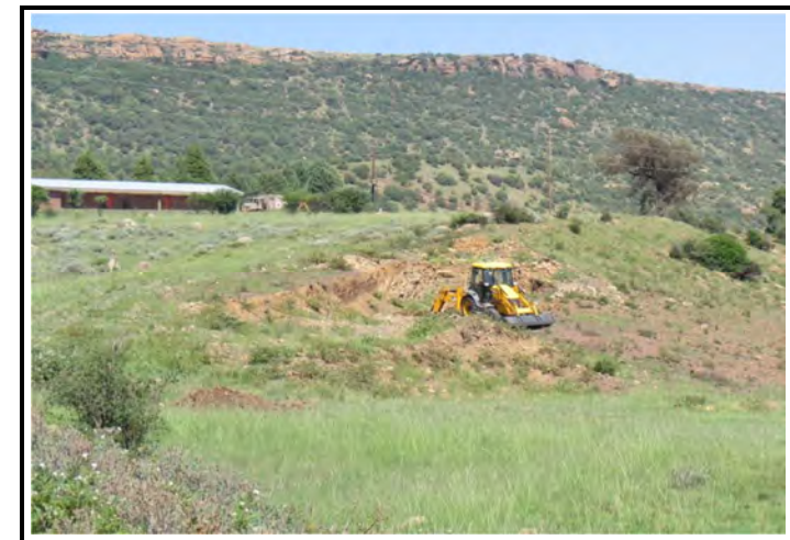
View of potential borrow pit target area - note proximity of existing structure
