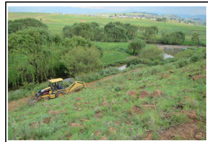
Typical view of potential borrow pit target area - note proximity of existing structure
