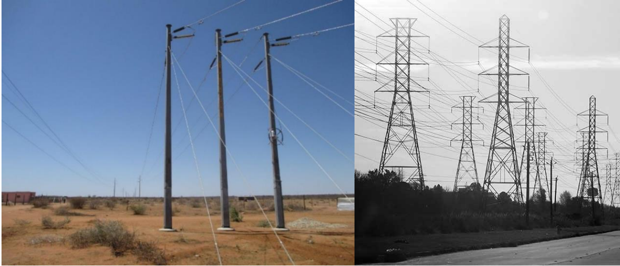
Figure 5-2: Left: Monopole pylons anchored to the ground with stays / anchors 18 . Right: Steel Lattice Pylons on a transmission line 19
