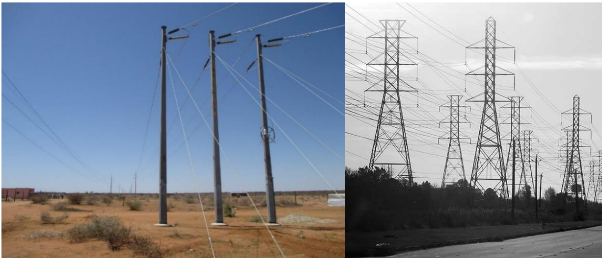
Figure 5-2: Left: Monopole pylons anchored to the ground with stays / anchors 18 . Right: Steel Lattice Pylons on a transmission line 19
