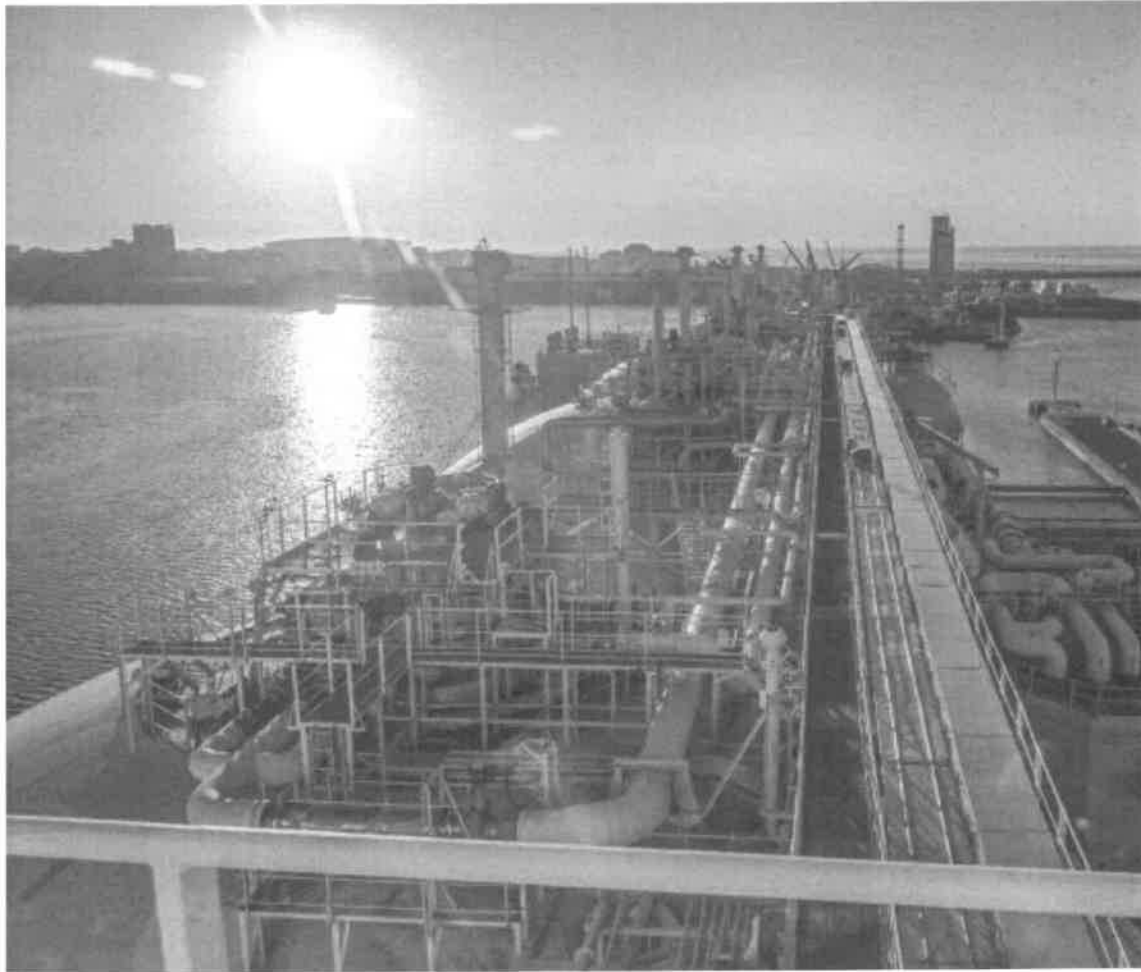
Tank pipework onboard the Karmol LNGT Powership Asia floating storage and regasification unit (FSRU), operated by Karpowership, via docked at Cape Town port in Cape Town, South Africa. Photographer: Dwayne Senior/Bloomberg via Getty Images
