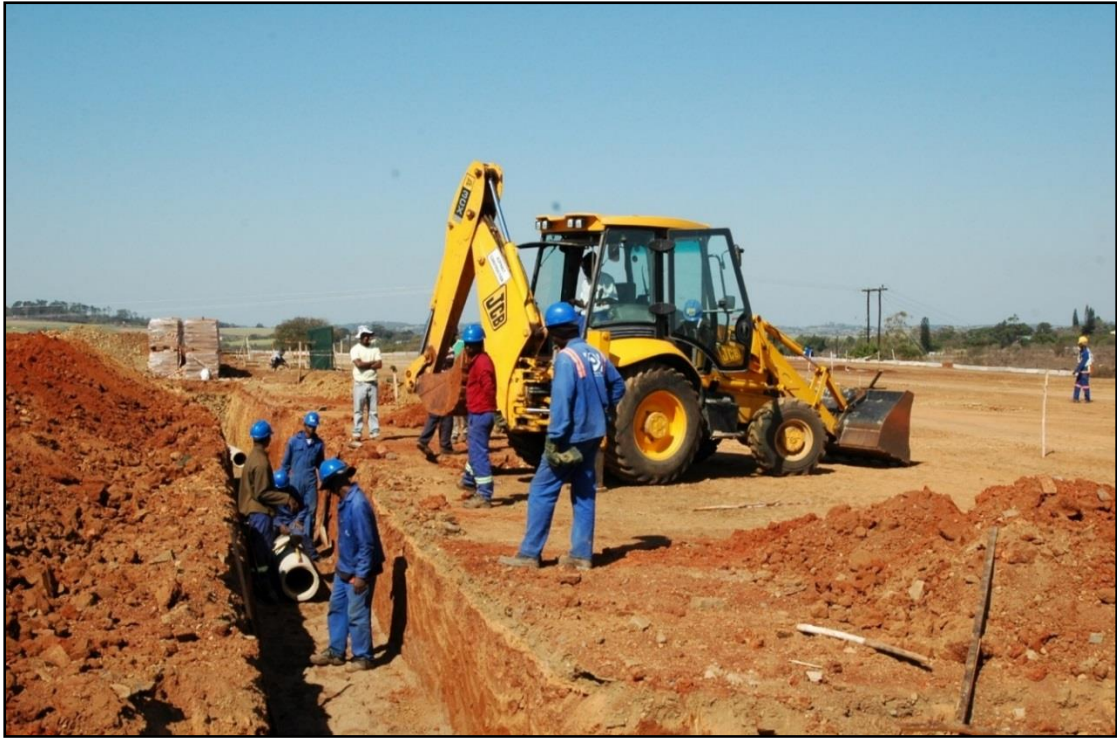
Plate 3: Construction of foundations and concrete works, including storm water drainage pipes, slabs, bund walls, a control room and a small building and storage area
