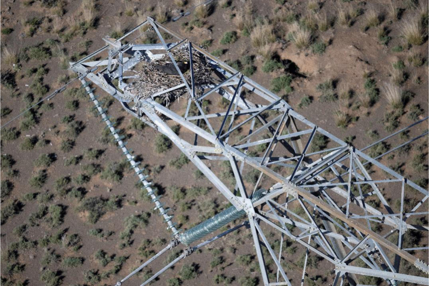
Figure 7: An active Verreaux's Eagle nest on existing HV powerlines within the assessment corridor
