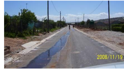
10. pipeline in road reserve – no crossing any road stormwater lines that drain to wetland
