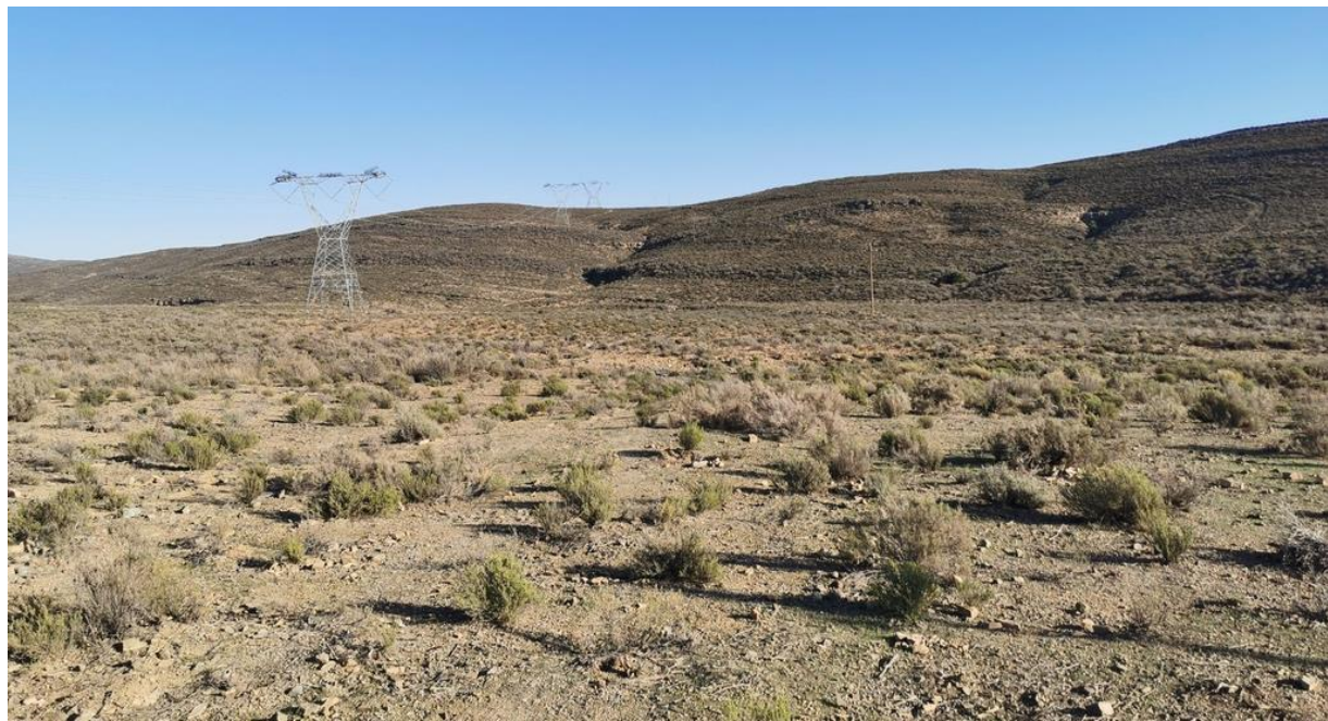
Figure 19: OHP route near Komsberg substation.
