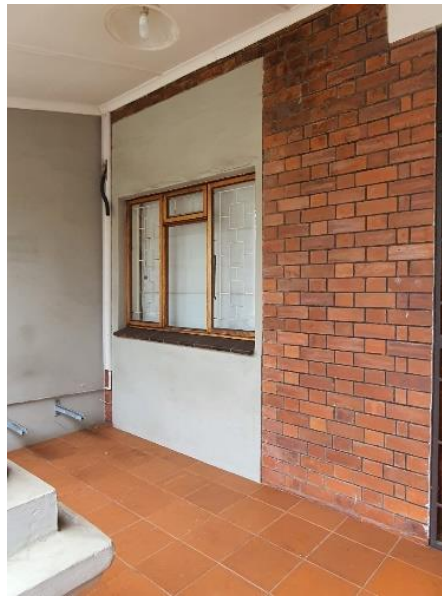
Inappropriate window addition
