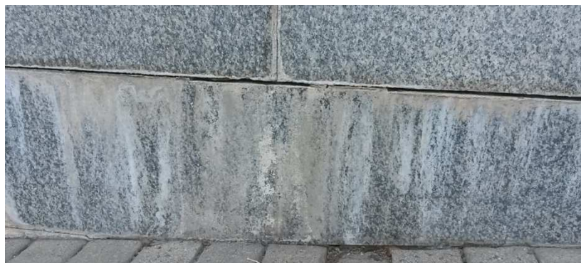
Photo 4.17: Localized efflorescence visible at bottom of planter
