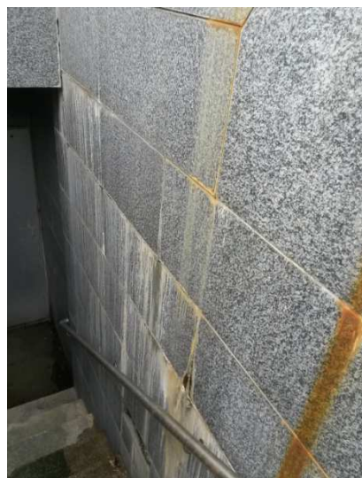
Photo 4.38: More visible efflorescence and corrosive staining on the same staircase.
