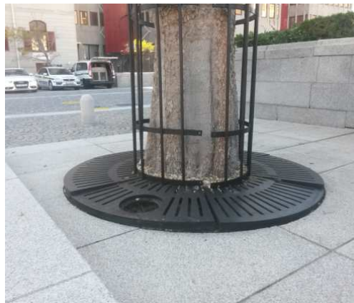
Photo 4.41: Tree close to Parliament entrance that has damaged the tree ring and also lifted granite pavers. Tree ring should be removed or modified to suite and granite pavers lifted to review extent of root growth, for trimming of roots and relaying of pavers. Investigate other trees as well
