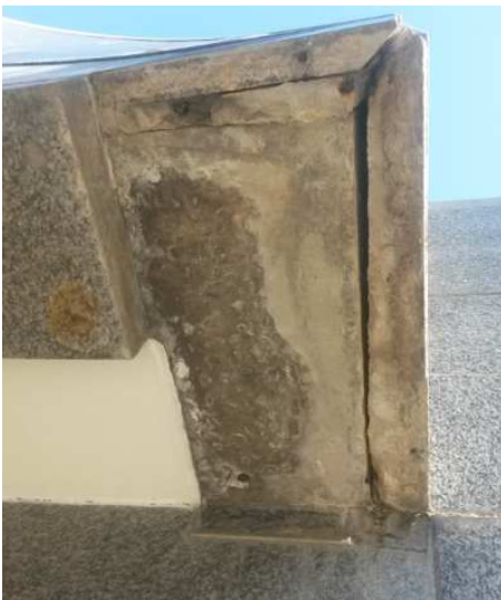
Photo 4.2 – Overhead granite panel that has fallen off. Could happen to other overhead panels as well.
