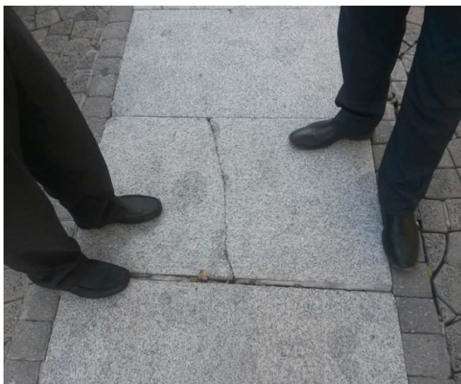
Photo 4.22 & 23: Granite slabs that have cracked in Parliament street
