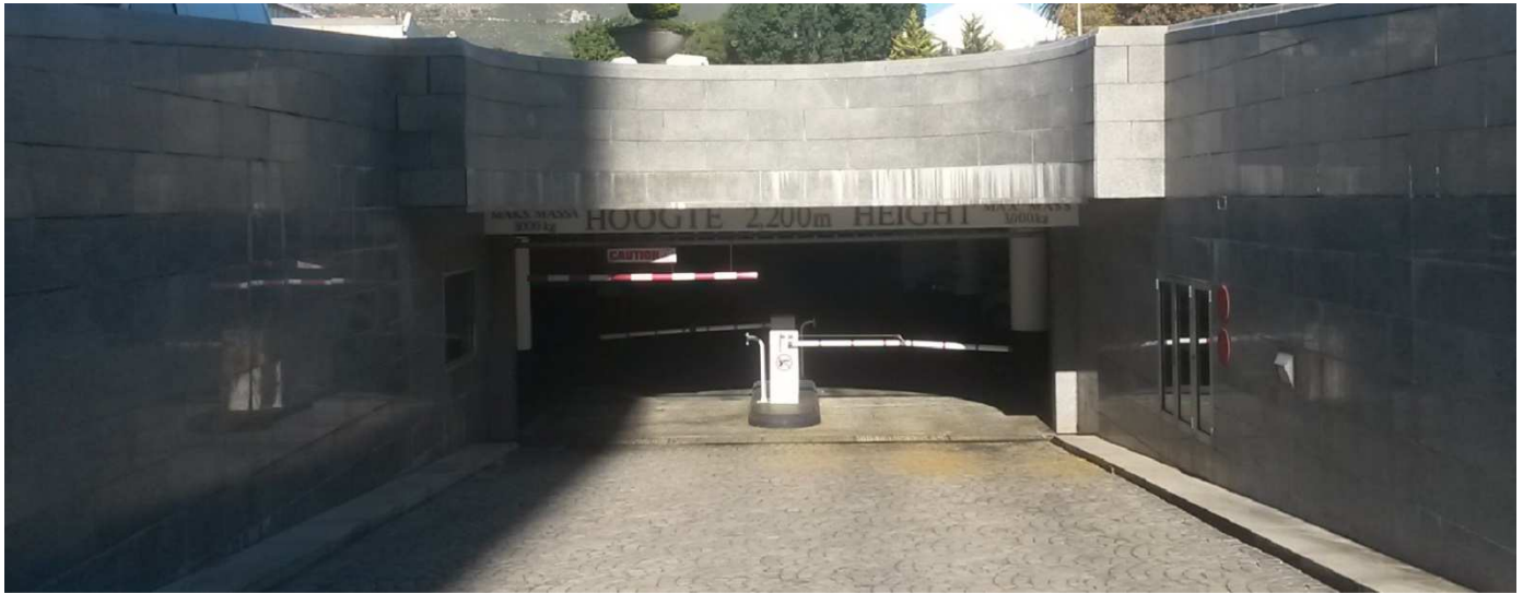
Photo 4.1: Efflorescence visible on curved granite element and also missing overhead granite panel on right hand corner.
