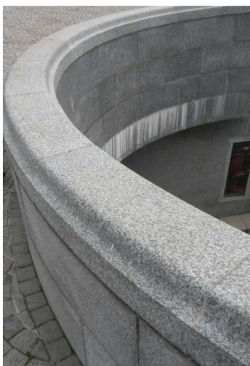
Photo 4.7: Curved granite entrance with concrete pavers at the top where water ingress through the granite elements occurs.
