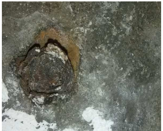
Photo 4.3 – Close-up of remnants of fixing anchor that is showing signs of corrosion.
