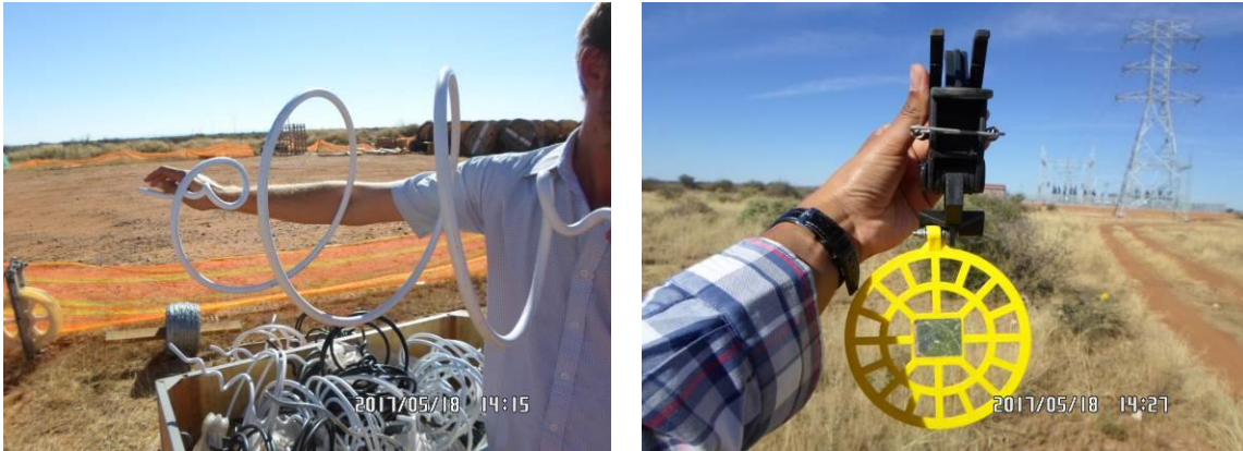
Figure 21: Examples of bird flight diverters to be used on the power lines: Double loop bird flight diverter (left) and Viper live bird flapper (right).
