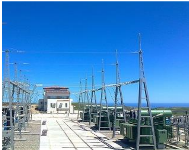
PLATE 1, BUS BARS ARE THE HIGHEST SUBSTATION ELEMENTS IN PICTURE
