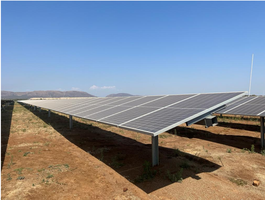
Photograph 1-1 Typical Photovoltaic Solar Energy Facility
