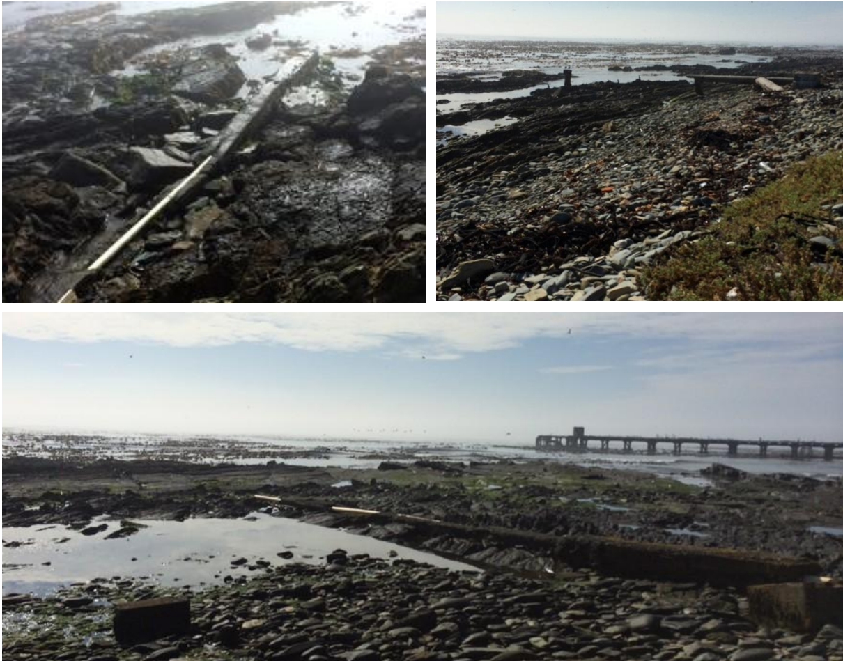
Figure 21: Some of the old sewage discharge pipelines discharging into the intertidal area on the eastern shore of Robben Island.
