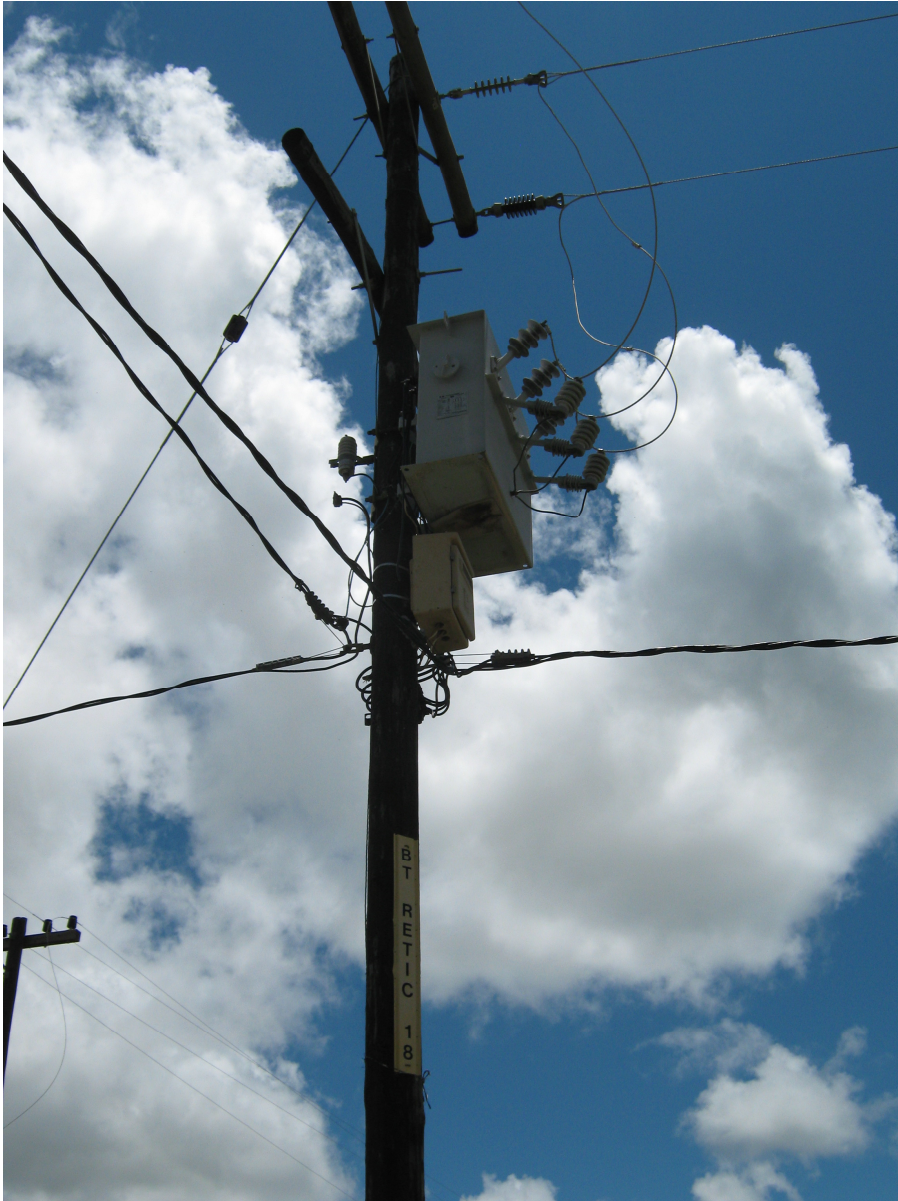
Nearest Three Phase Power Supply
