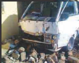
Rubble tells the story of a taxi that ploughed through the wall.
