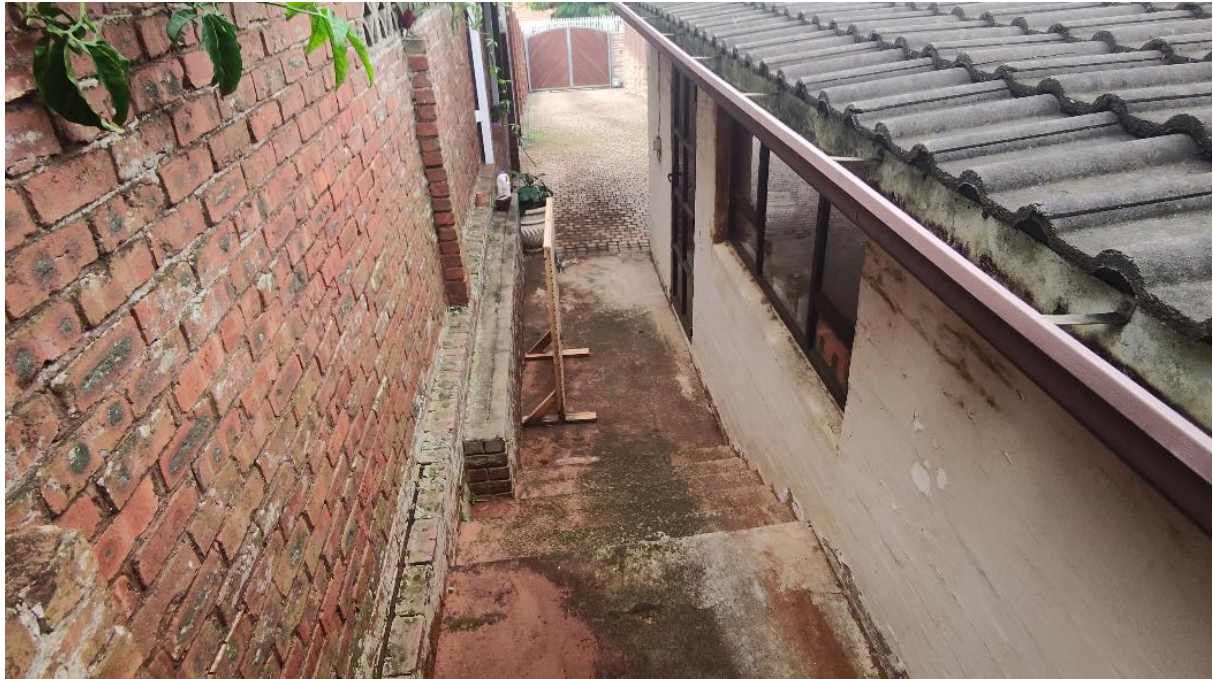
A5. Image illustrates the service passage between the garage and boundary wall
