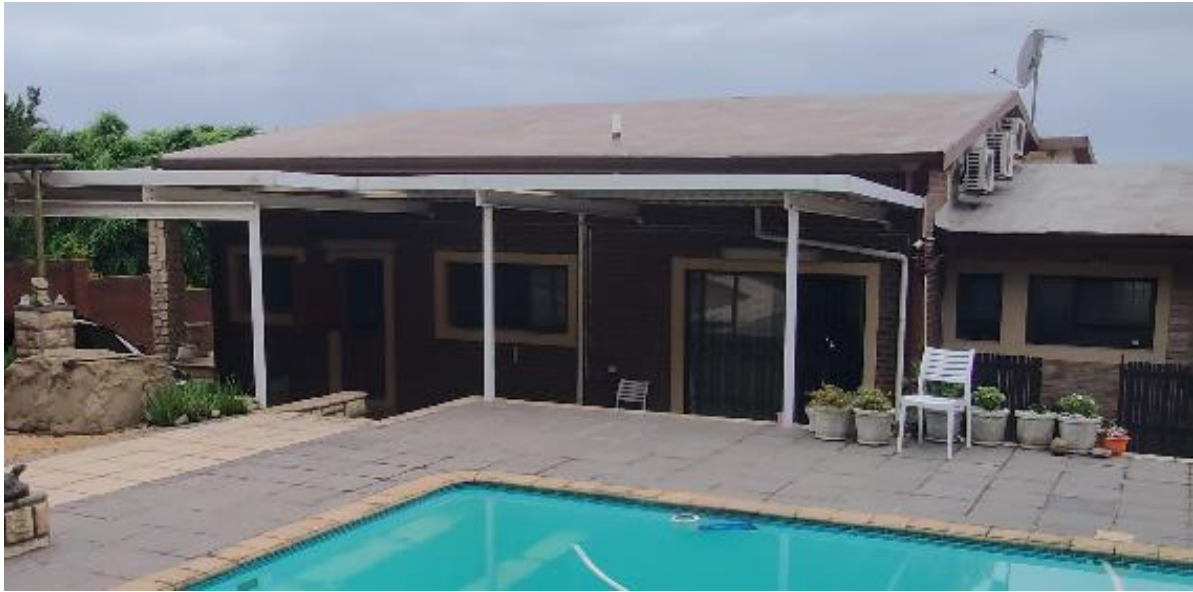
Figure 7 (page 7). Image illustrates the current poor condition of the roof sheeting which is to be replaced in accordance to the attached plans.
