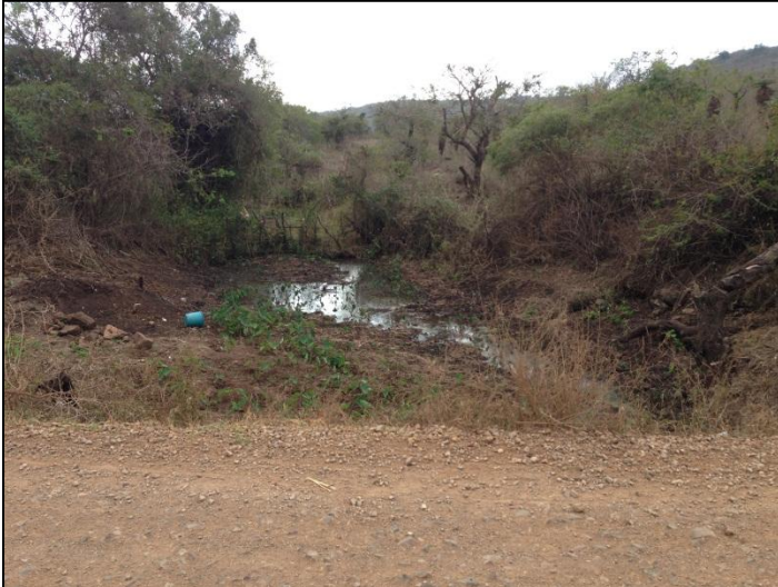
Figure B4 Watercourse Crossing on the Raw Water Rising Main en route to WTW.
